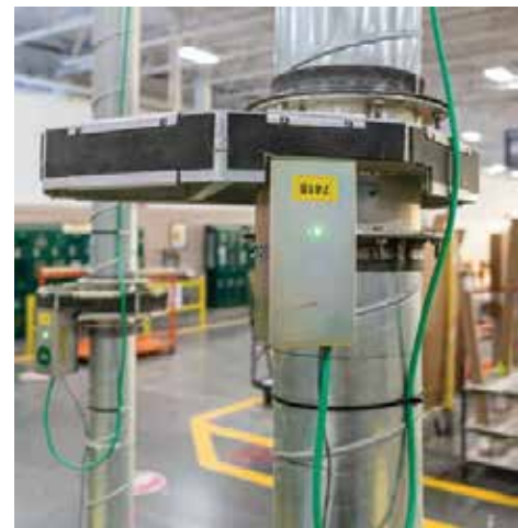
Automatic gate on dust collection pipe.
