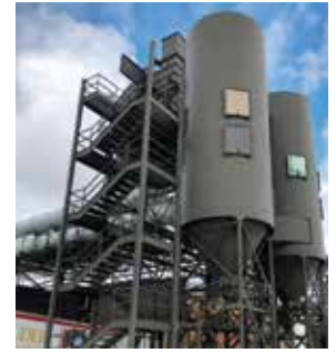
Dust collection filter house
