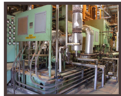
Steam flows through the turbine to generate power.
